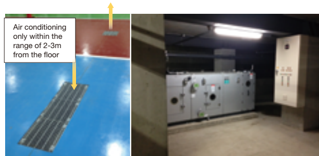
Air Conditioning Equipment Installed in the Pit and Vents on the Floor
