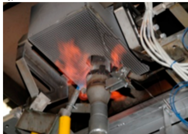
Example of Thermoelectric Power Generation for Carburizing Furnace
