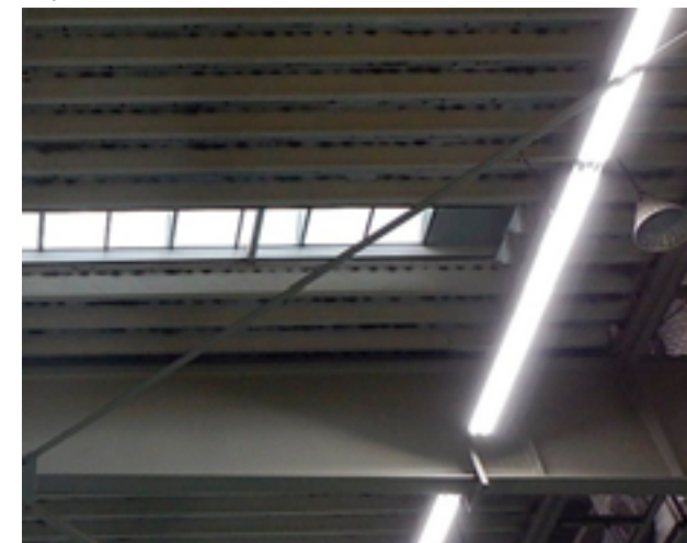
Ceiling lighting and modulated LEDs
