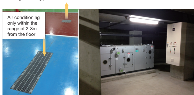
Air Conditioning Equipment Installed in the Pit and Vents on the Floor
