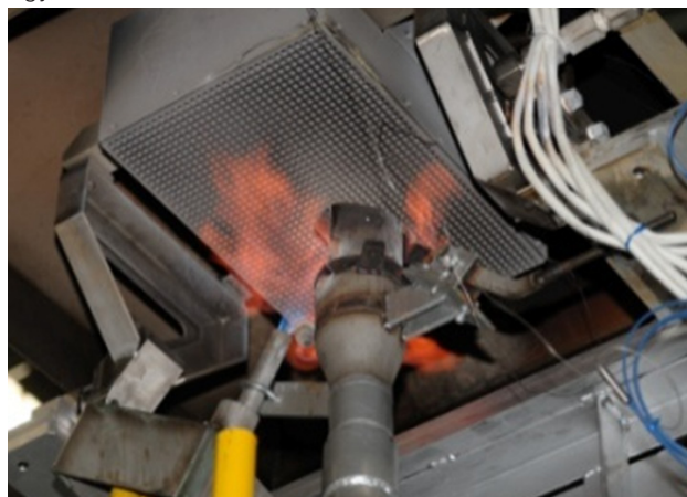
Example of Thermoelectric Power Generation for Carburizing Furnace
