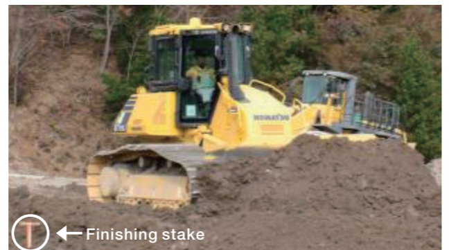
Construction in a manual operation in which finishing stakes are checked visually (previous procedure)
