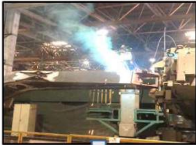
Measures against soot while welding: KSC (Jining, Shandong) (Fence that prevents soot from spreading, using a dust collector)
