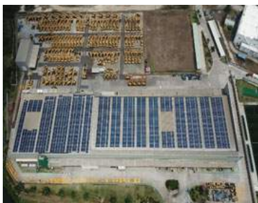
FY2018: Installed solar roof(920.7 kW)
