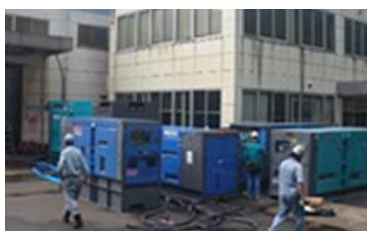
Examples of recovery support (lending of power generators and assistance in machine centering)
