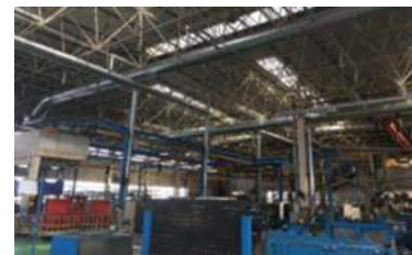
An example of measures to meet regulations in China (Daikyo Machinery Shandong Co., Ltd.: Installation of a welding fume dust collector and exhaust air ducts)
