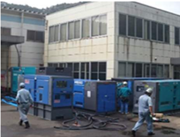
Disaster recovery support (lending electric generators)
