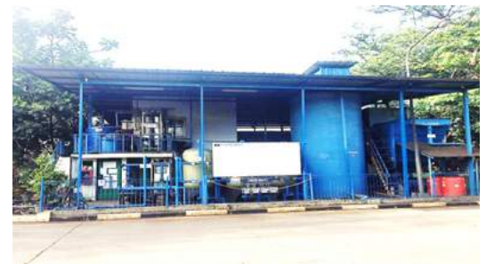
Komatsu Indonesia's wastewater recycling facility
