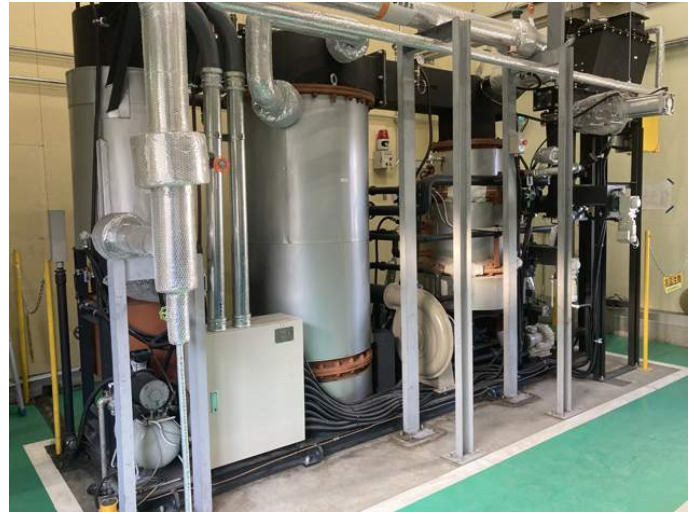
Ibaraki Plant biomass boiler
