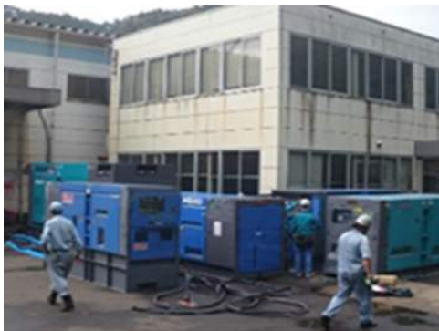
Disaster recovery support (lending electric generators)
