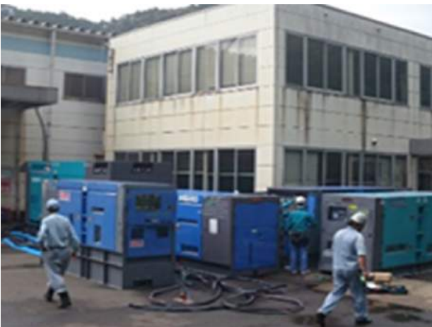
Disaster recovery support (lending electric generators)
