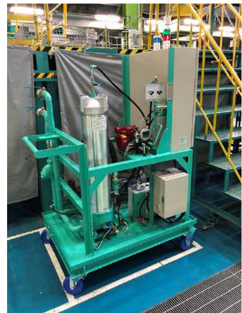
Oil Purification System
