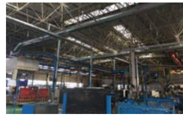
An example of measures to meet regulations in China (Daikyo Machinery Shandong Co., Ltd.: Installation of a welding fume dust collector and exhaust air ducts)
