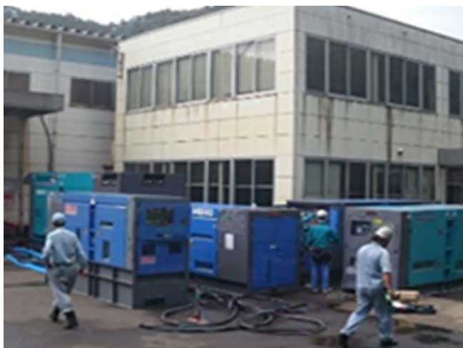
Disaster recovery support (lending electric generators)
