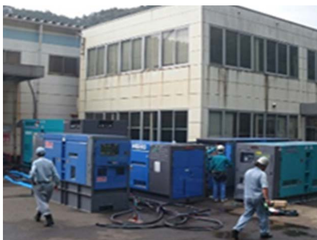
Disaster recovery support (lending electric generators)
