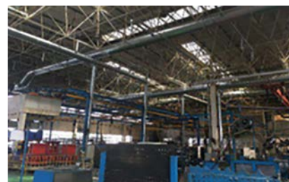
Example of measures taken to comply with regulations in China (Daikyo Machinery Shandong Co., Ltd.: Installation of a dust collector and exhaust ducts for welding fumes)
