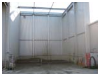
A station for washing vehicles with high walls to minimize the impacts on the surrounding community of the sound and water during washing (Fukuoka Nishi branch of Komatsu Rental Japan Ltd.)
