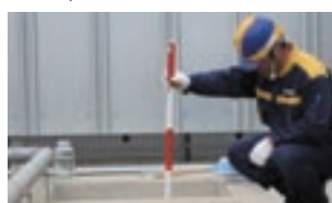
Inspecting the oil-water separator at a vehicle washing station (Komatsu Rental, Koriyama)
