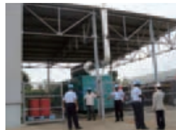
Measurement for exhaust gas emissions from the electrical generator (in Komatsu India Pvt. Ltd.)
