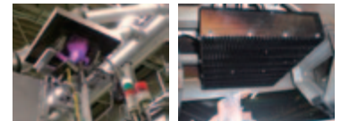
Thermoelectric Unit (the Awazu Plant)
