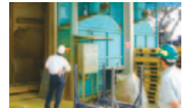
Paint Booth and Dust Catcher
