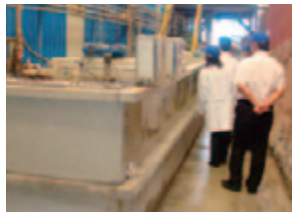
Water Treatment Facility for Waste from Electrostatic Coating
